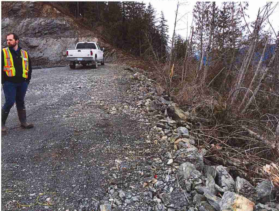
Photograph 6. – Perched fill along top of north slope of quarry viewed to the west.
