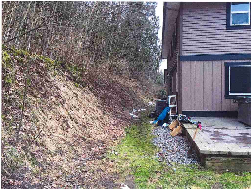
Photograph 20. – Approximate 3 m high slope immediately upslope of residence. Approximate 400 mm high concrete foundation wall along south side of residence.
