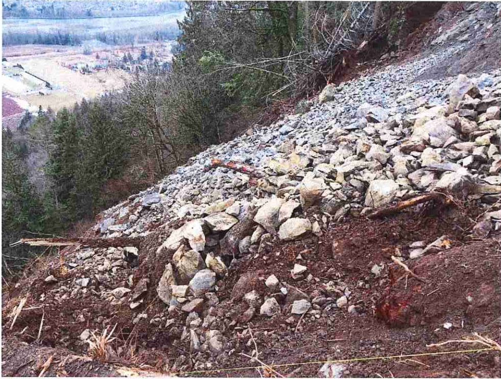
Photograph 1. – Loose cobbles and boulders immediately below initiation zone.
