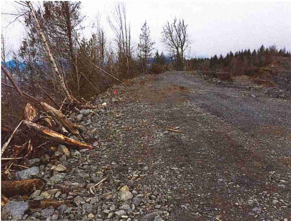
Photograph 7. – Perched fill along top of north slope of quarry viewed toward the east.
